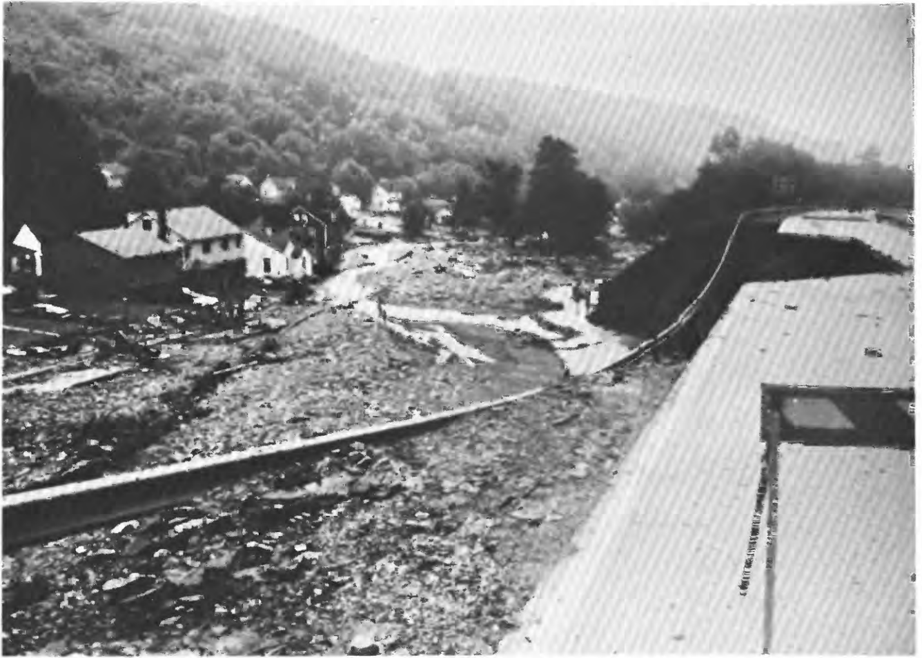
FIGURE 32. - Eastbound lanes of State Highway 56, near Johnstown's eastern corporate boundary, undermined by floodwaters from Solomon Run (Pennsylvania Air National Guard photograph).
