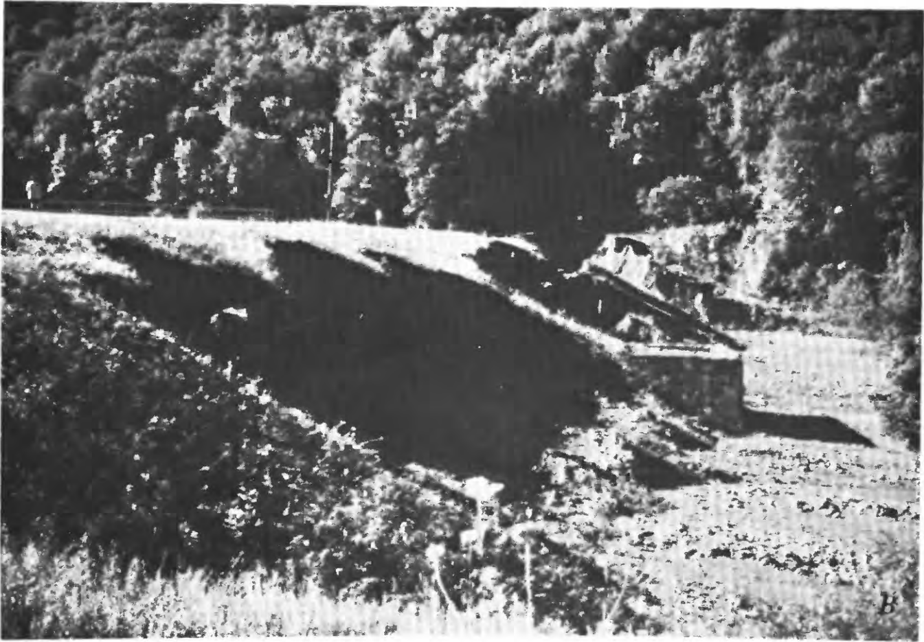
FIGURE 27.—Laurel Run Dam. A , The left photograph shows the view looking downstream through the breach. (Pennsylvania Air National Guard photograph). B , The right photograph shows the eroded downstream face of the dam. The breach is at the far end. (U.S. Geological Survey photograph.)
